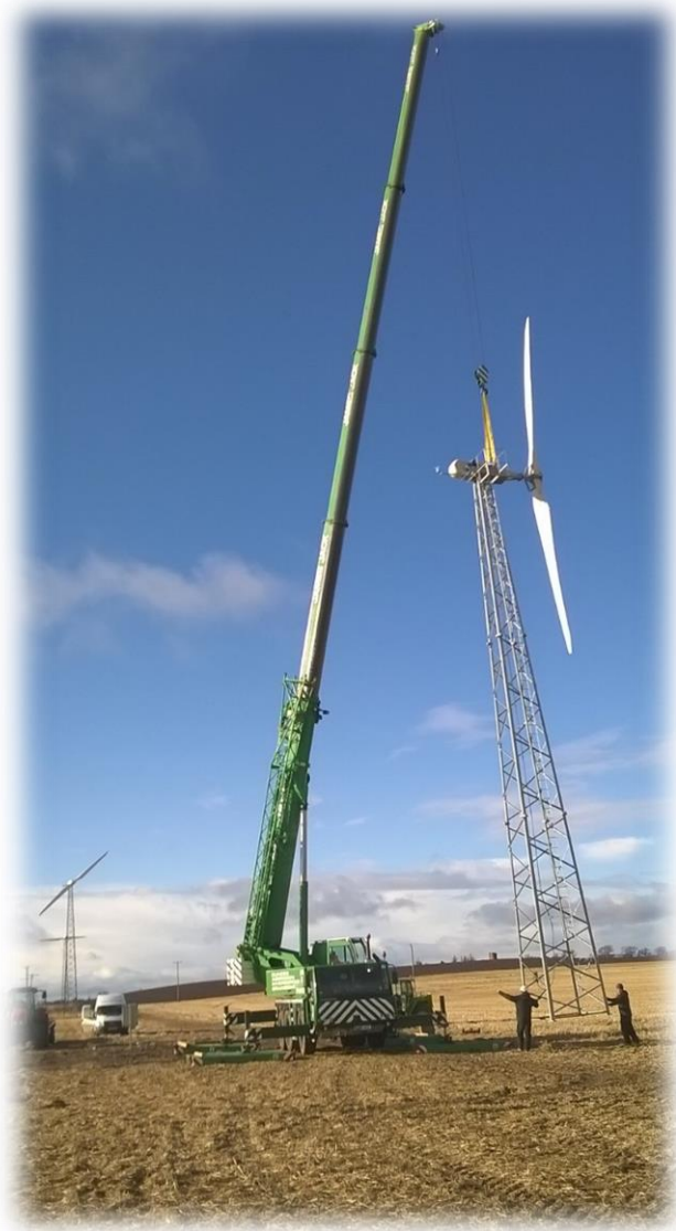
Installing the Gaia 11kw wind turbines at the Agrico UK head office
